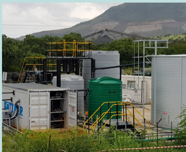
DCM 450 cubic metre per day water treatment plant
